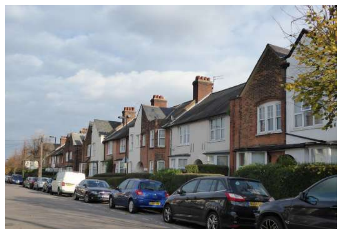
Painted brickwork disrupts cohesion of this terrace
