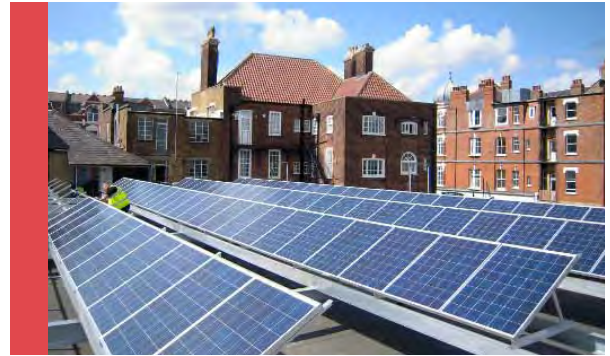
Community-owned solar array on Marks & Spencer roof, Muswell Hill Broadway
