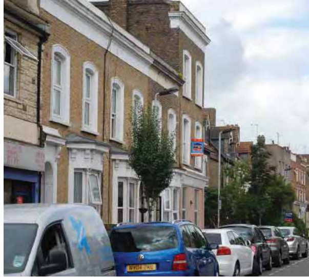
Poor conditions of existing buildings
